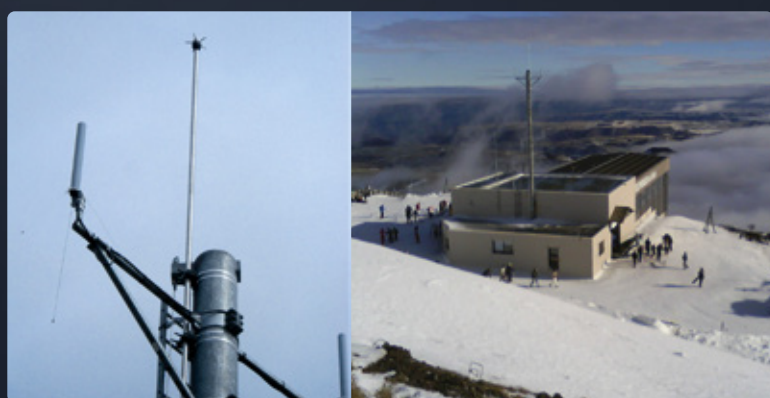
ESE air terminal in extreme climatic conditions
